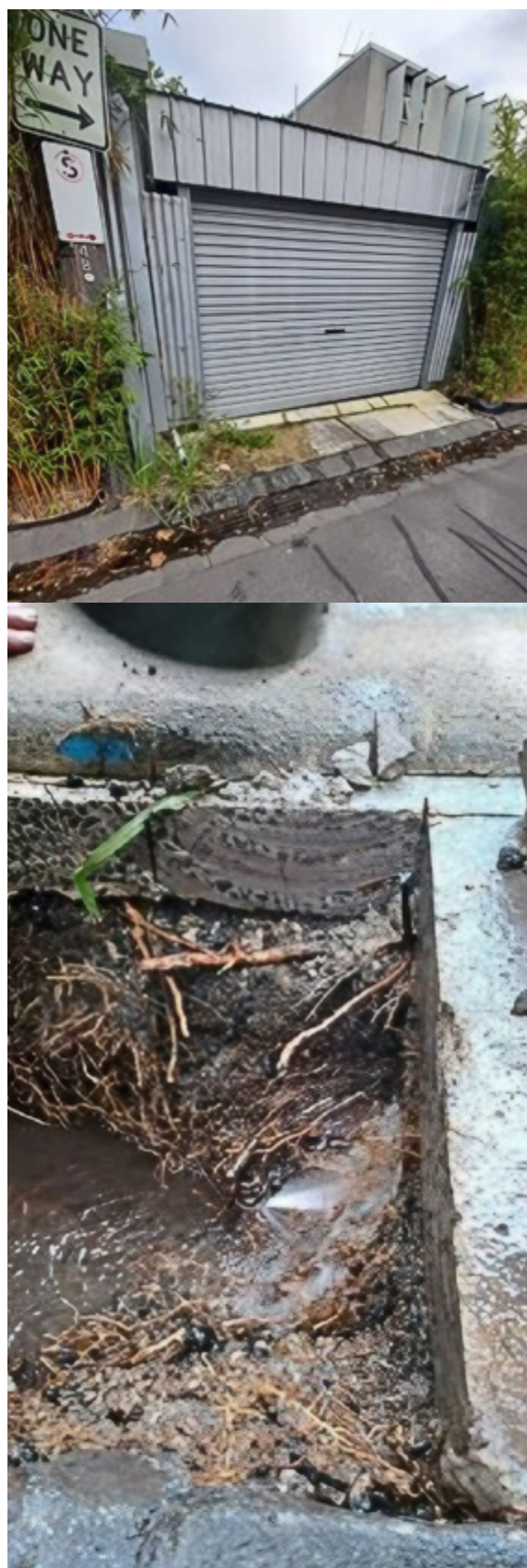
Figure 3 Pictures associated with a particular leak.
